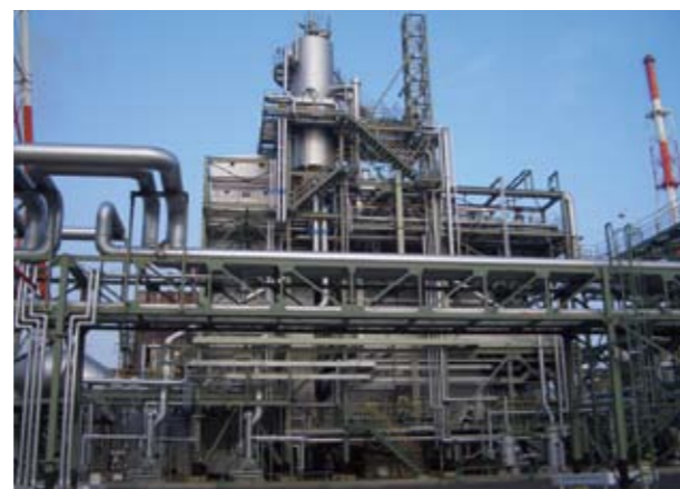
Mizushima Plant / Exhaust gas re-burning system
